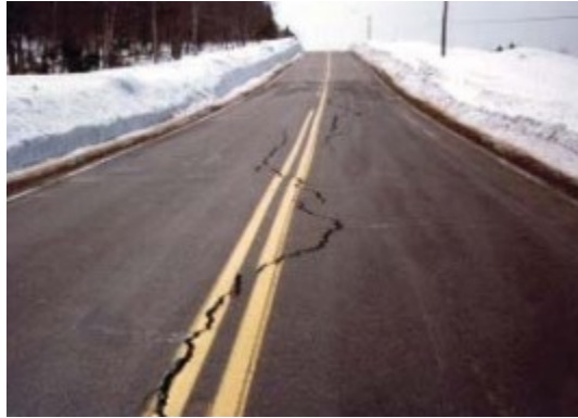
Figure 12 – Fissure de gel (MTQ, 2011)
