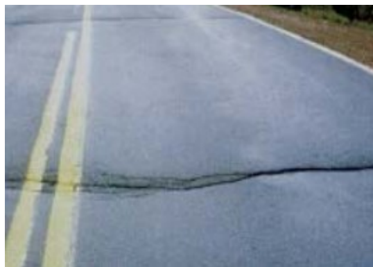
Figure 9 – Fissure transversale (MTQ, 2011)
